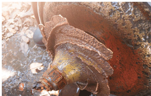
Fig. 7 – Strongly corroded pump rotor used in sewage treatment plants.
