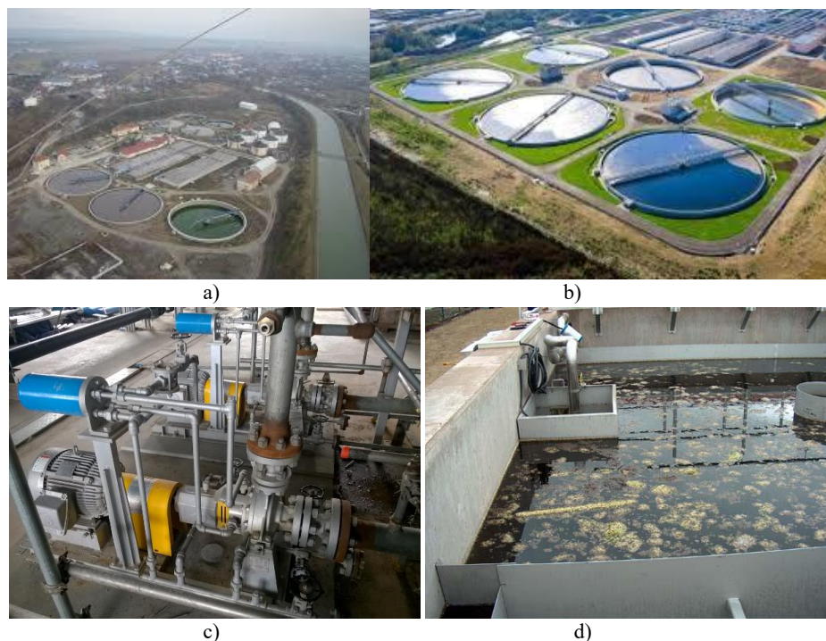
Fig. 1 – Treatment plants for industrial and domestic wastewater and their operating elements: a) wastewater treatment plant - spatial view; b) Piatra Neamț industrial wastewater treatment plant; c) action elements; d) baths for chemical cleaning of wastewater.
